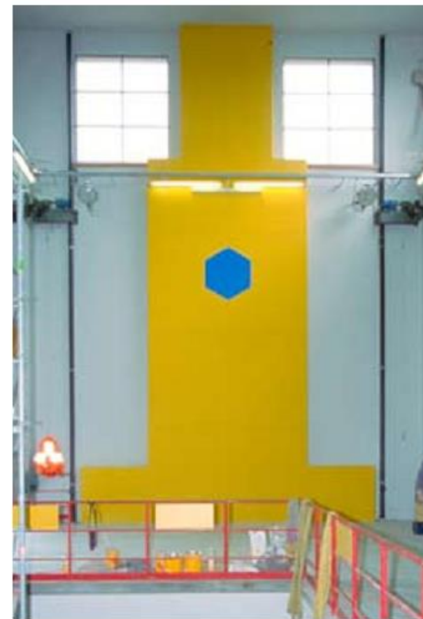
New reinforced concrete structural wall from the inside of the east facade of the assembly shop.
