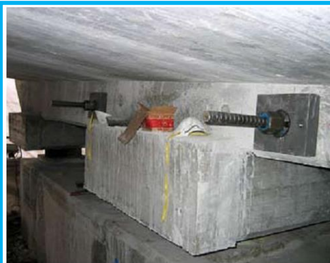
Tightening together both bridge halves at the original expansion joint in the middle of the bridge.
