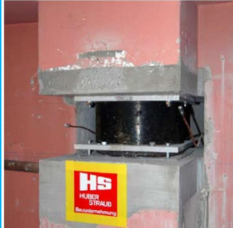
Installation of a seismic elastomeric bearing under a column in the outside wall of the basement.
