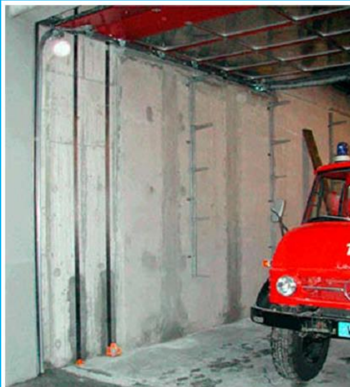
Two post-tensioned CFRP-strips on the inside of the gable wall (Truffer et al. 2004).
