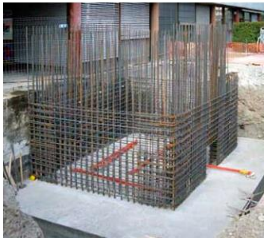
Steel reinforcement in the basement and foundation of the new stairway towers.
