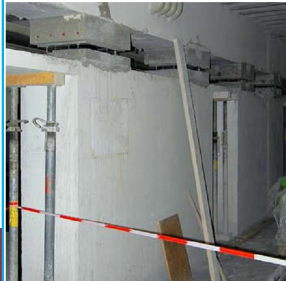
Sliding bearings were installed under the column-free inner region of the ground floor.
