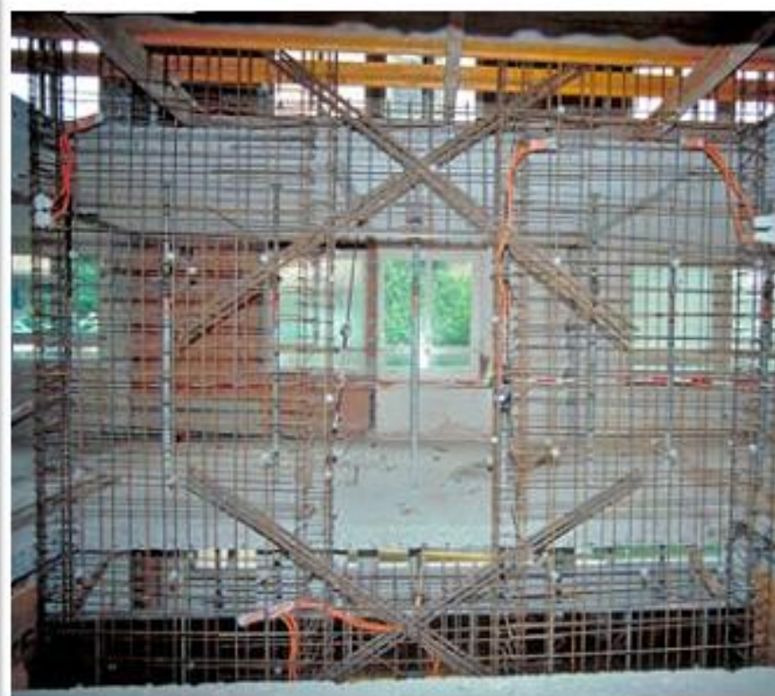
Reinforcement of the new coupled reinforced concrete structural walls in the ground floor level with diagonal bundled bars in the coupling beams.
