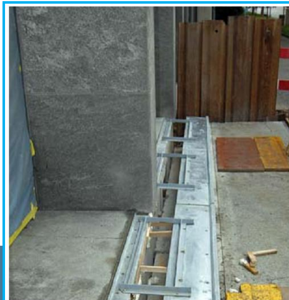
An expansion joint was installed around the building to permit the free, horizontal movement on the new seismic isolation bearings.
