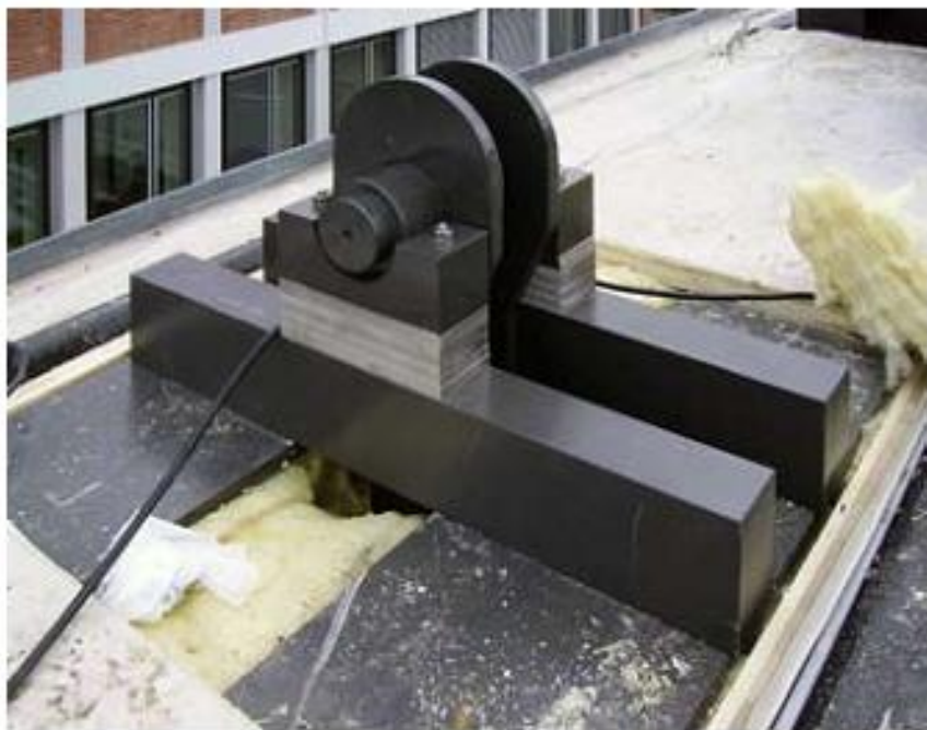
Upper anchorage of the carbon fiber tension rod on the roof from where the post-tensioning occurs.
