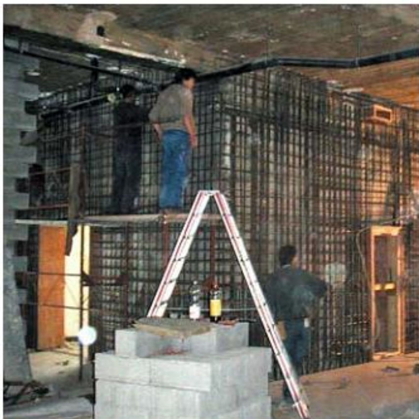
Installation of the reinforcing bars of the new reinforced concrete walls in the ground floor level.
