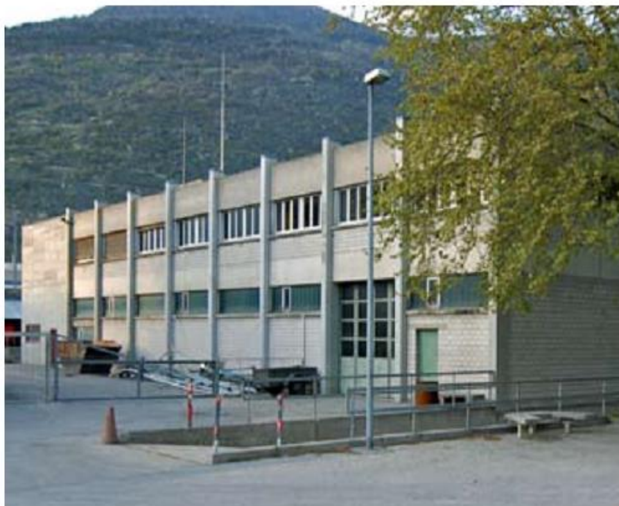
The longitudinal facade of the rear of the fire station stiffened by the reinforced concrete structural wall at the left end.
