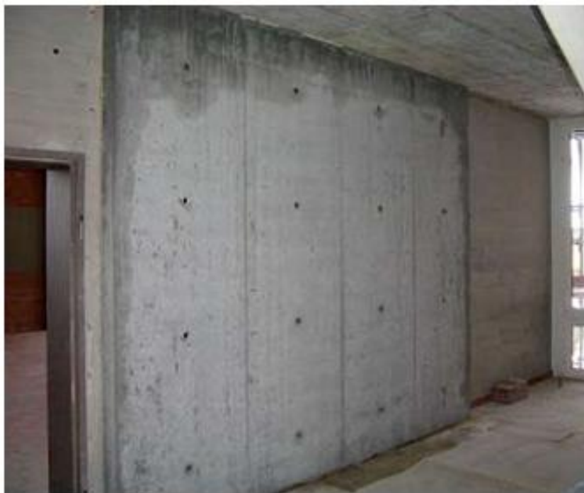
Strengthening of an existing reinforced concrete wall with a 15 centimetre thick double wall.
