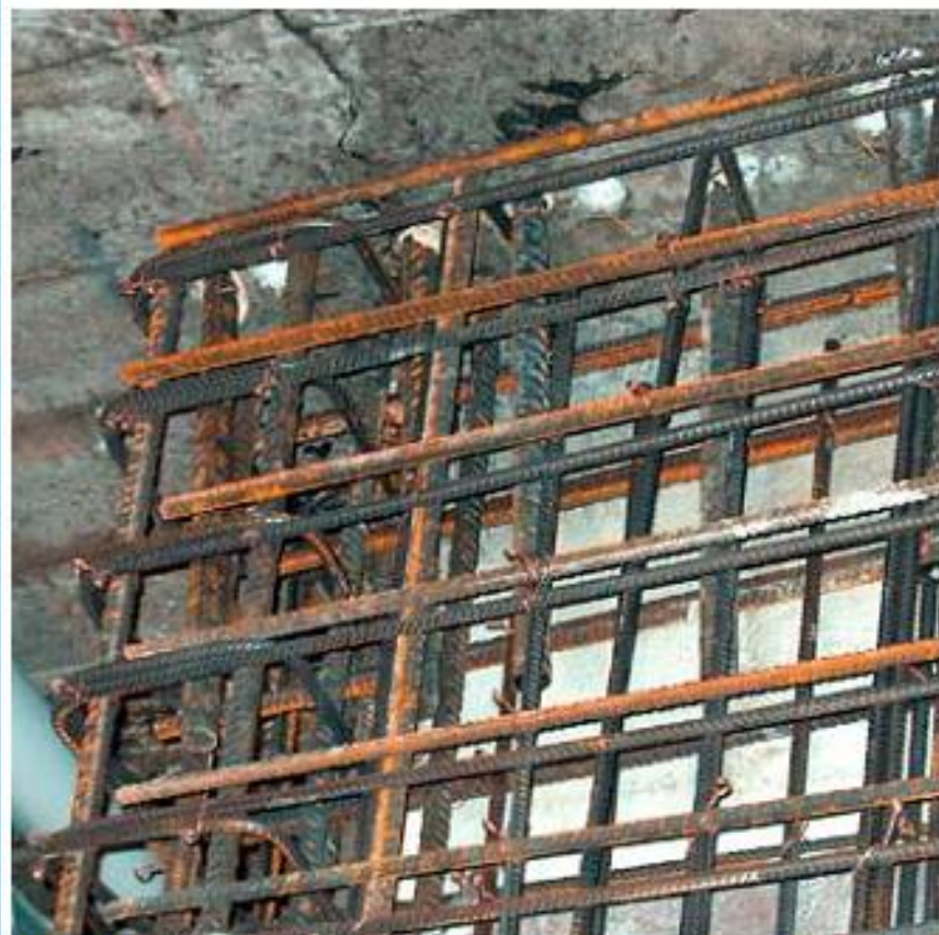
Detail of the connection of the new wall's reinforcing bars with the existing floor (Garcia-Vogel 2005).
