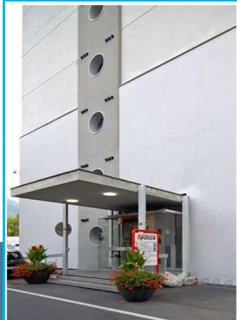
Transverse facade of the existing building showing the anchorages of the tension strands visible on the outside at each storey level.
