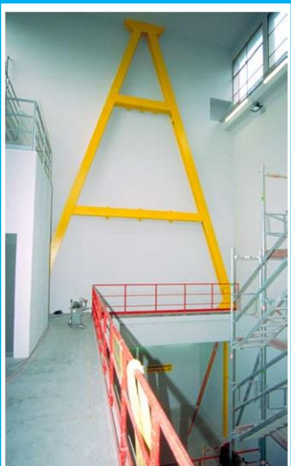
New A-shaped steel frame in the ground floor level of the west facade and new steel plates in the basement.
