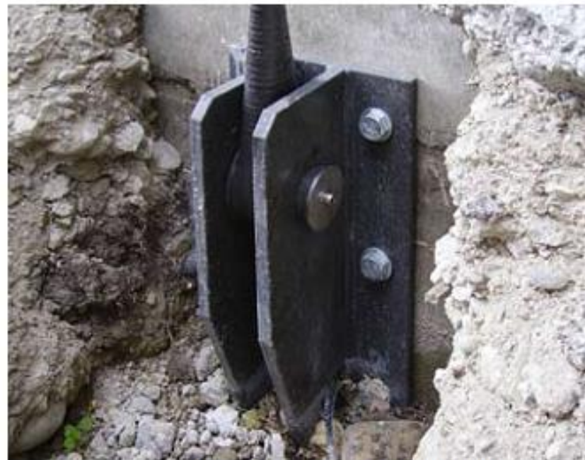
Lower anchorage of the carbon fiber tension rod on the side of the basement wall.
