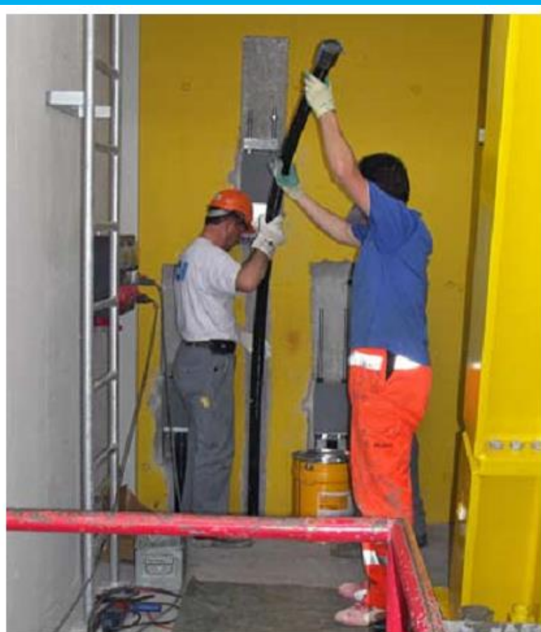
Threading of the CFRP-strips to the anchorage of the new reinforced concrete structural wall.
