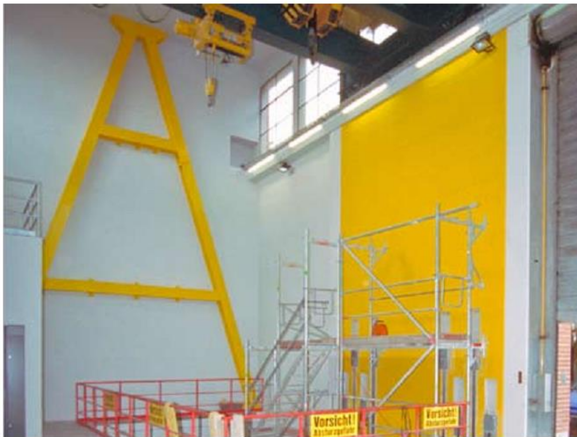
New A-shaped steel frame on the west facade and new reinforced concrete structural wall on the north facade of the assembly shop.
